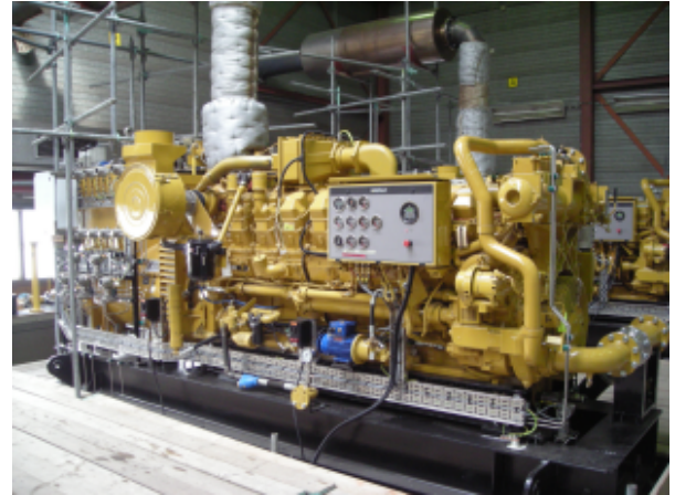
Figure 4: Gas engine during operational testing
