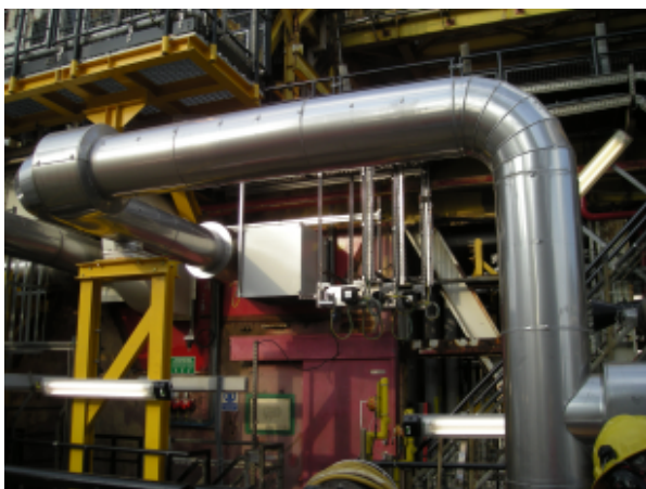
Figure 12: Engine exhaust duct acoustic lagging
