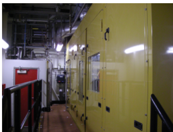
Figure 8: Acoustic enclosure and access walkway
