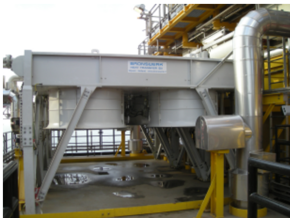
Figure 6: Fan coolers on cantilever platform
