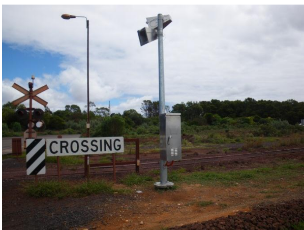
Figure 2. Wayside horn installation
