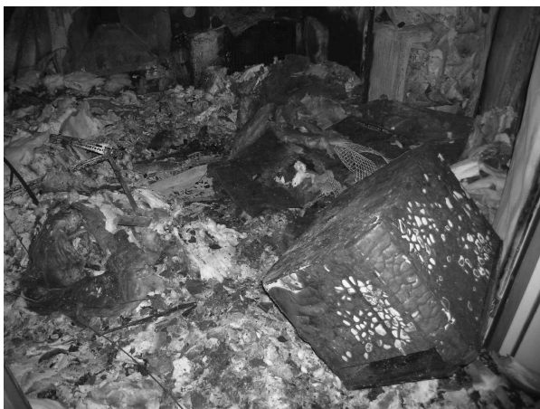
Figure 3. Anechoic Room after the fire
