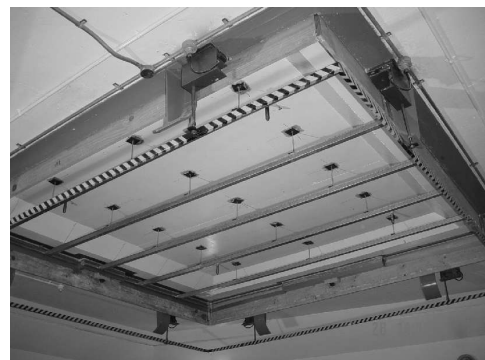
Figure 5. Array of battens suspended from a concrete floor before the installation of the ceiling panel.
