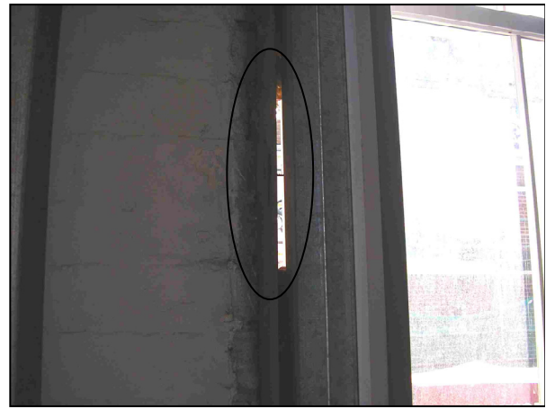
Figure 2 shows the extent of the gaps around the window frame.
