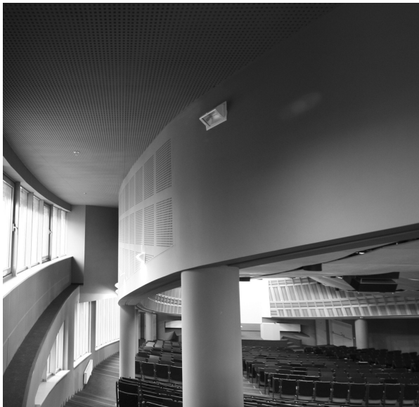
Figure 10. Arrangement of acoustic materials in side aisle area: view on perforated plasterboards on the ceiling and the outside of suspended partition ring
