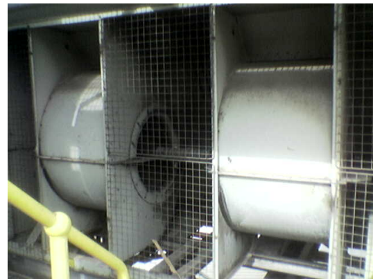
Figure 2: Cooling tower fan
