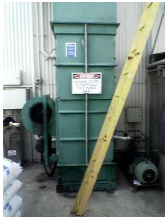
Figure 3 : Fibreglass cooling tower and fan
