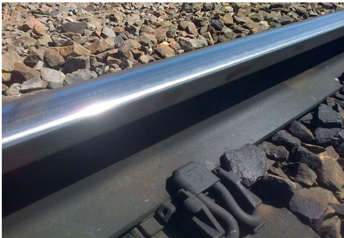
Figure 5 – The LOW rail on a tight curve showing a clear running band on the gauge corner. The gauge corner and face would be rusty in the absence of wheel contact.
