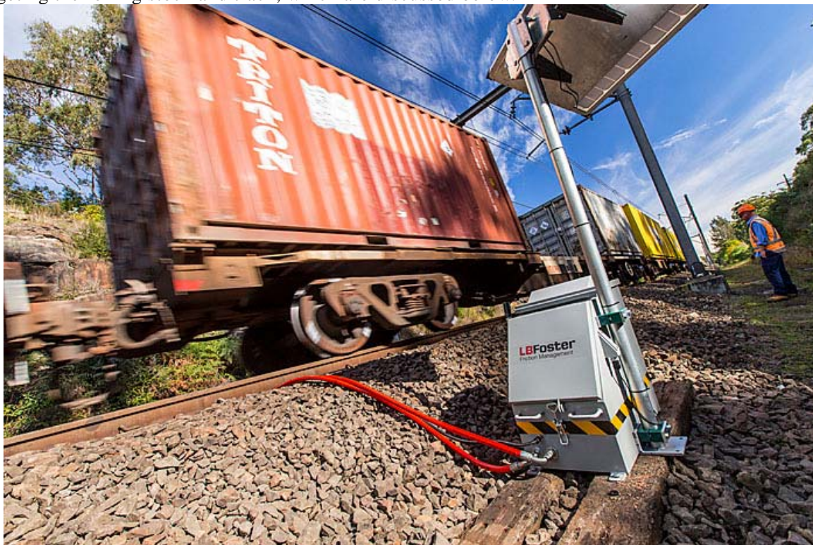
Figure 3 – TfNSW installed modern electronic lubricators at several curve noise sites
