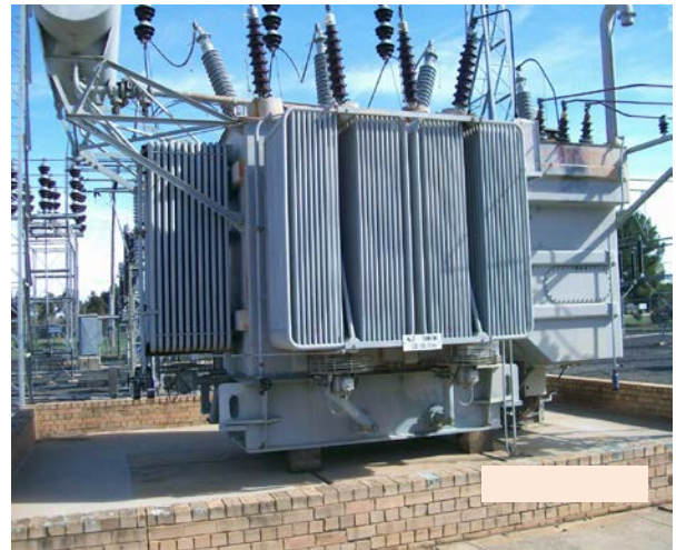
Figure 1 Typical substation transformer
