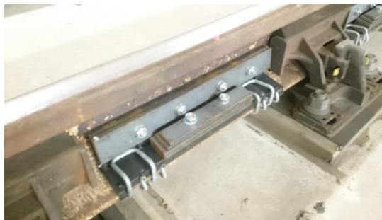
Figure 1 Installed rail damper, Perth Tunnel 6, 30 August 2016.
