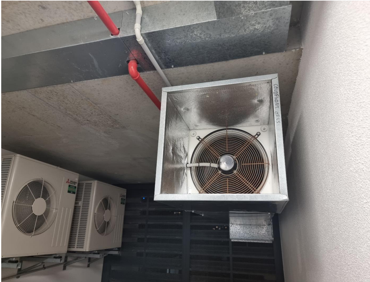
Figure 3 – Exhaust fan at the plant room of a high-rise building in central Gold Coast
