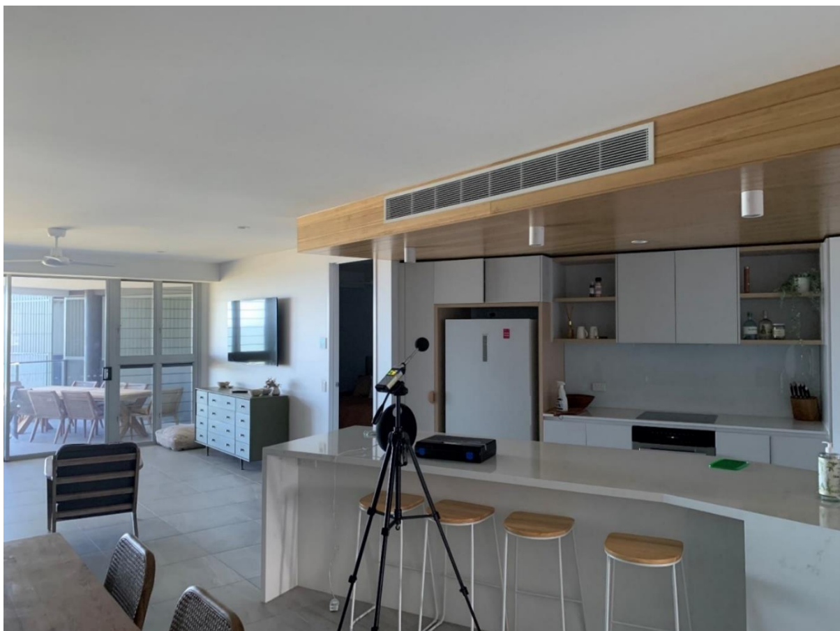
Figure 2 – Bulkhead in the kitchen with return air grill facing the dining area
