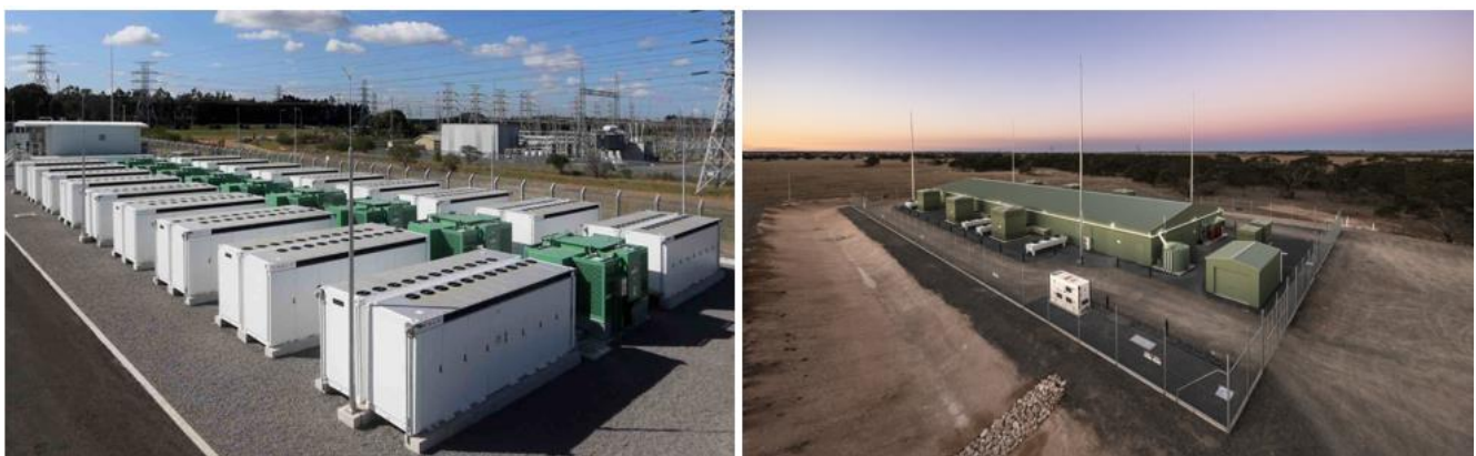
Figure 2 – Outdoor centralized (right (RenewEconomy, 2021)) and indoor centralised (left (ElectraNet, 2024)) Large-Scale Solar BESS
