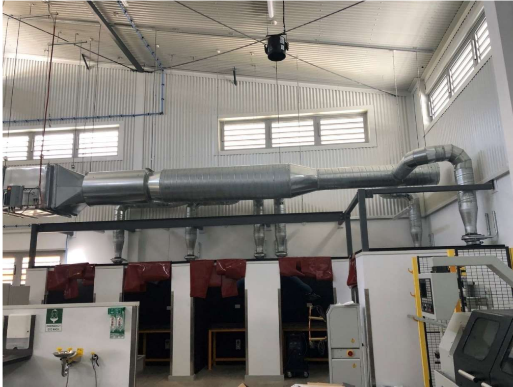
Figure 6 – Senior engineering workshop with welding booths and fume extraction system
