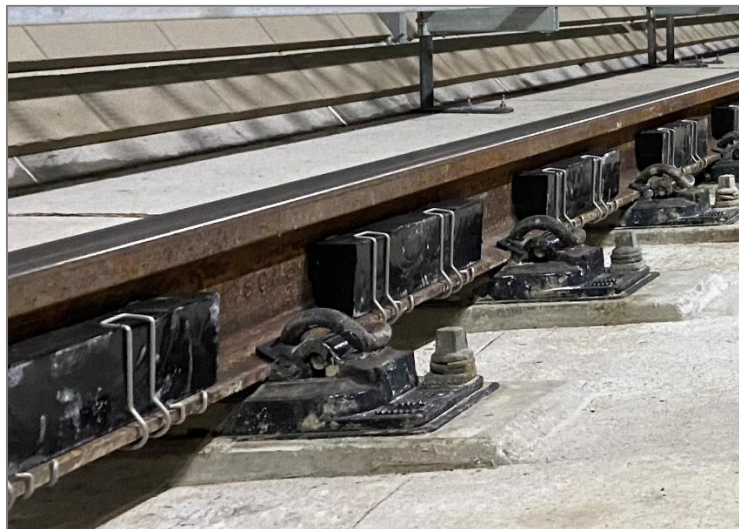
Figure 2: Rail web dampers fitted to Sydney Metro, 2022 (Image credit Pyrotek Pty Ltd)
