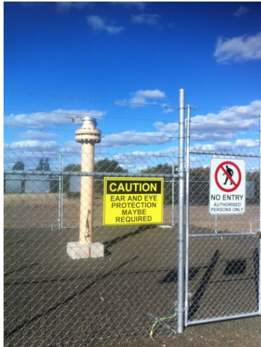
Figure 1 Blowdown valve arrangement
