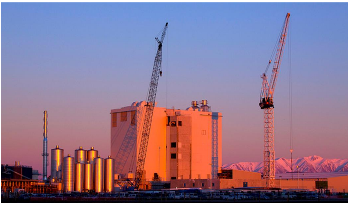
Figure 2 – Fonterra Darfield dryer 2 under construction with dryer 1 in background (image courtesy Fonterra)
