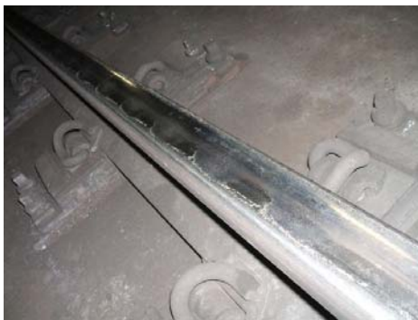
Figure 7. Photograph of the corrugated inner rail of the Down North Shore track
