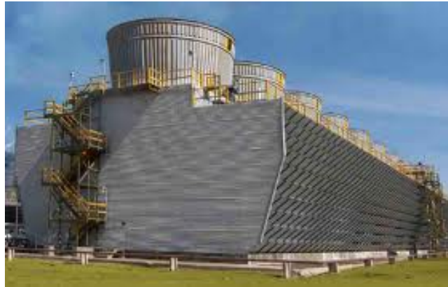
Figure 21: Typical industrial cooling towers cooled using axial fans with static regain systems.
